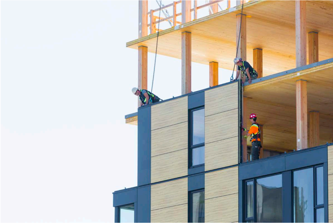
Figure 6. Construction of the Brock Commons student residence in Vancouver (UBC), the tallest cross-laminated timber (CLT) building in the world at 53m high. In many countries building regulations still limit the heights of timber buildings based on outdated regulations. Photo source: https://www.naturallywood.com/
