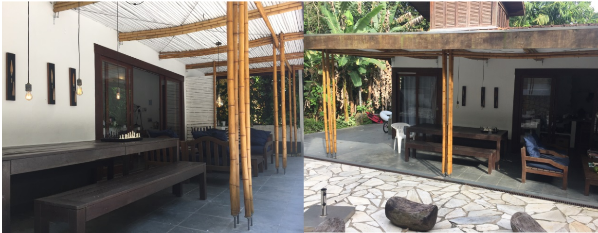
Figure 6.73. Finished veranda with a light buckling in the middle. 2016.
