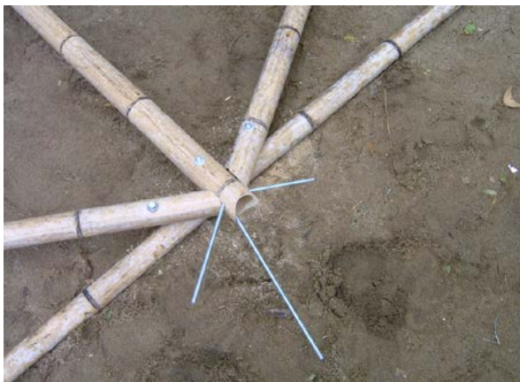
Figure 6.42. Fish mouth joints in the truss. 2006.
