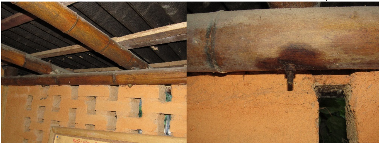
Figure 6.56. Fungi and mold on horizontally positioned bamboo members in a poorly ventilated area. 2017
