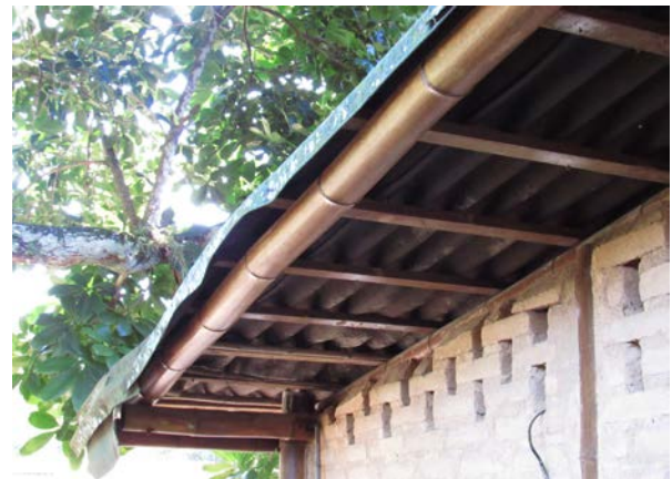
Figure 6.67. Inferior quality corrugated sheets. 2017.
