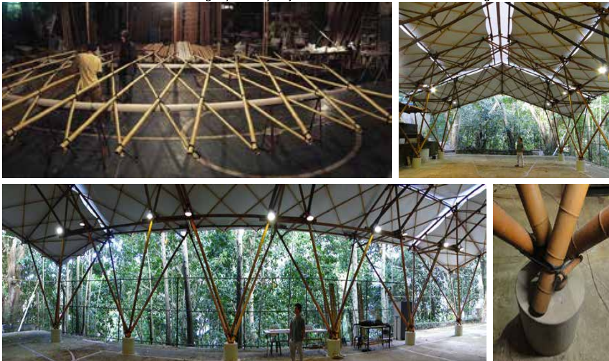
Figure 3.14. Pantograph grid shell structure. 2016. Retrieved from: Prefabricated bamboo structure and textile canvas pavilion (p.183, 186) by M. Seixas, K. Ghavami and J. Ripper. Copyright Journal of International Association for Shell and Spatial Structures.
