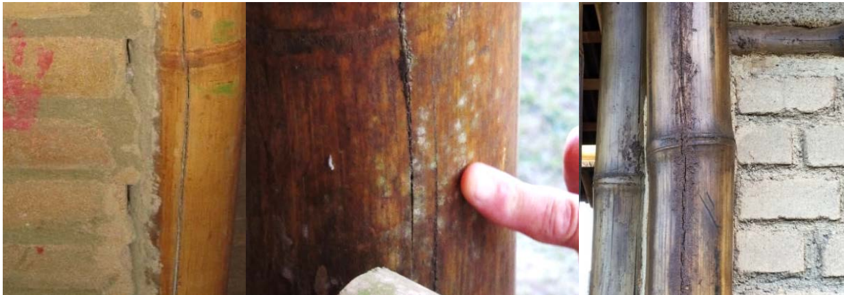
Figure 6.58. Cracks that pose no structural problem but need to be adjourned. 2017.
