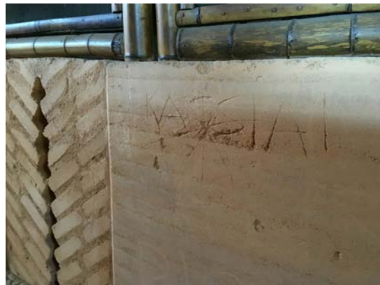
Figure 6.61. Vandalized rammed earthen wall. 2017.
