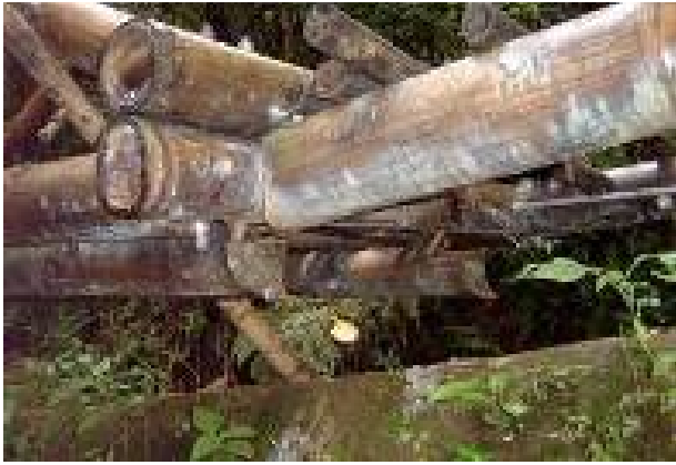
Figure 6.11. Mold where there is little ventilation due to high humidity level. 2005.
