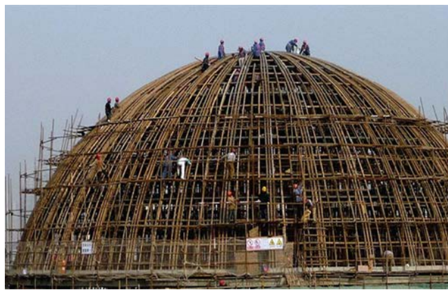
Figure 2.4. Indian Pavilion at Expo 2010 Shanghai China. Retrieved from Building with Bamboo (p.133) by Gernot Minke. 2012. Basel, Birkhäuser. Copyright Birkhäuser.
