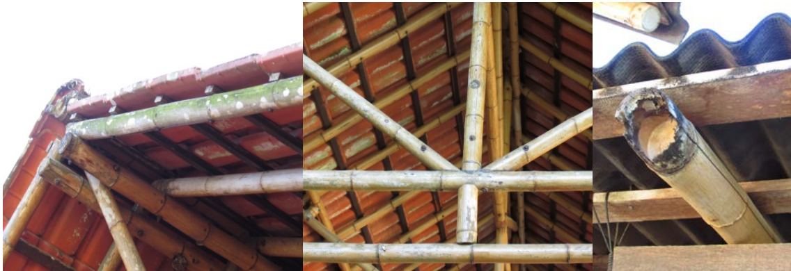
Figure 6.53. Affected bamboo on the front truss closest to the sea. 2017.
