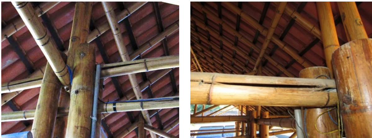
Figure 6.59. Cracks that do pose a structural problem and need to be resolved. 2017.
