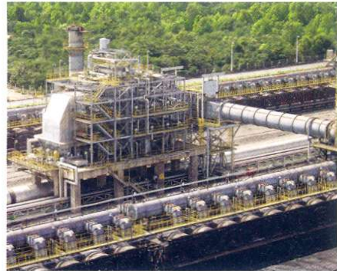
Figure 4. One of the heat-recovery boilers
