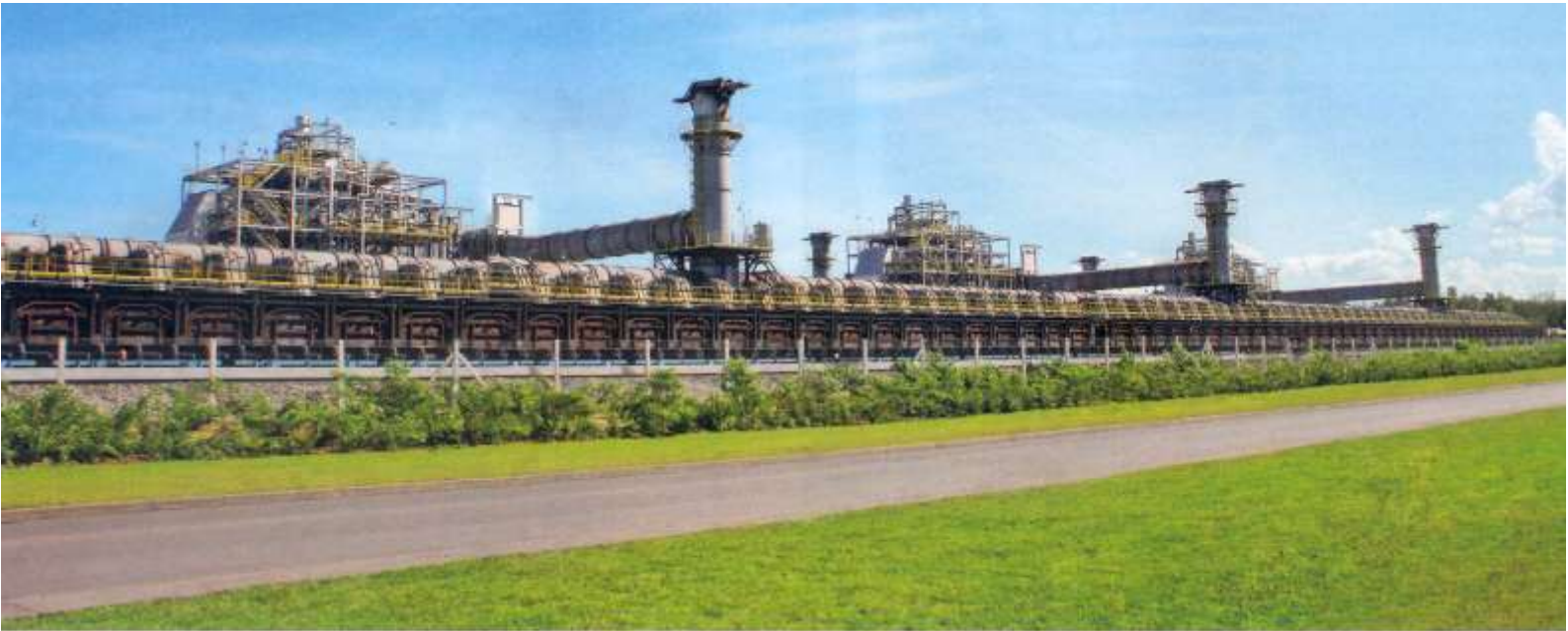
Coke oven battery with three heat-recovery boilers
