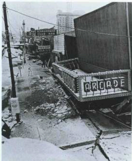
Earthquake, 4th Ave., Anchorage, Alaska. Photo by Steve McCutcheon, Alaska Pictorial Service.
