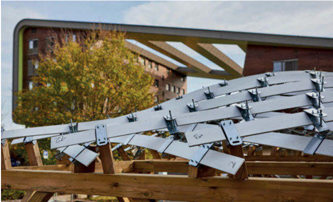
Fig. 4: The pseudo-geodesic pavilion, made of 100 mm GFRP lath at 60^\circ with a unique Z-connector. (Picture: Charlene Yves)
