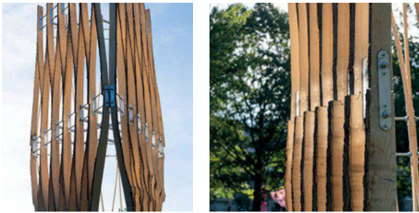
Fig. 10: Left: connection between panels C and D; Right: splice connection. (Photos by Cynthia Kuo)
