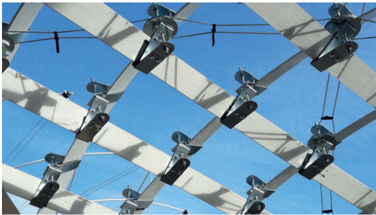
Fig. 9: The standard nodes developed in this study and bracing system. Laths cross-section: 100 × 8 mm.
