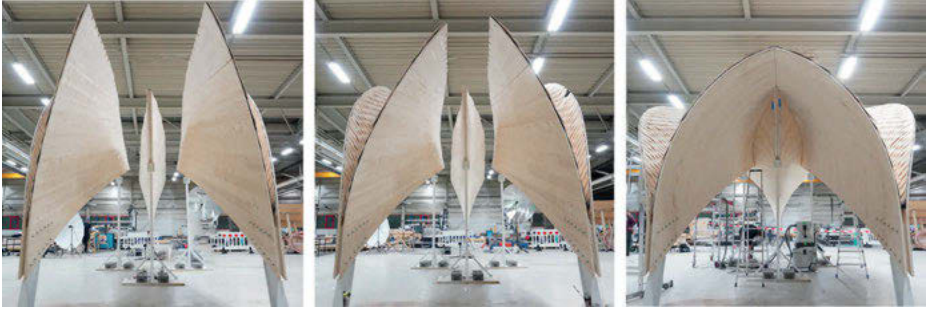
Fig. 5: In situ self-shaping of the bilayer timber building components. Starting flat in a vertical configuration with high MC in the active layer, during shaping, and after full shaping and interlocking.
