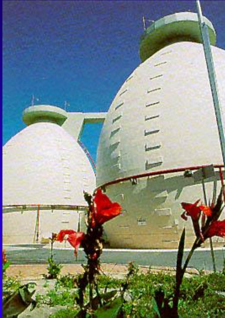
Municipal Sludge Digesters
