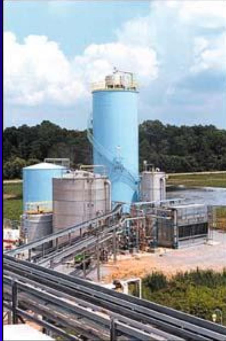
Kraft Paper Mill Foul Condensates, Alabama
