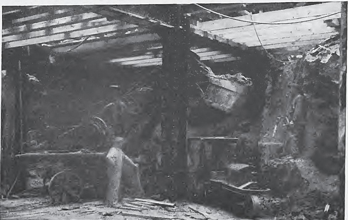
Hudson Department Store, Detroit. Making the general cellar excavation after the caissons, columns, and cellar walls had been installed in pits and the steel work erected.
