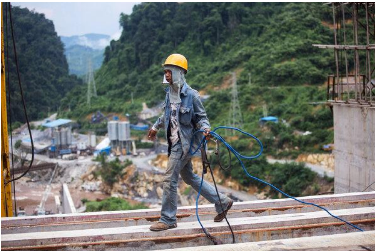
China has been supporting dam construction in southeast Asia, including the Nam Tha 1 hydropower plant in Laos. Credit: Taylor Weidman/Bloomberg/Getty
