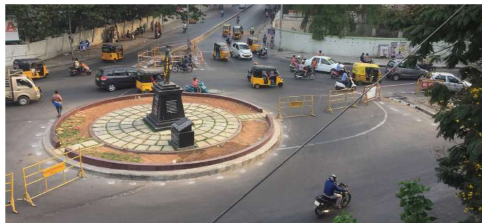
Fig. A roundabout and traffic islands under construction on Pantheon Road in Chennai.
