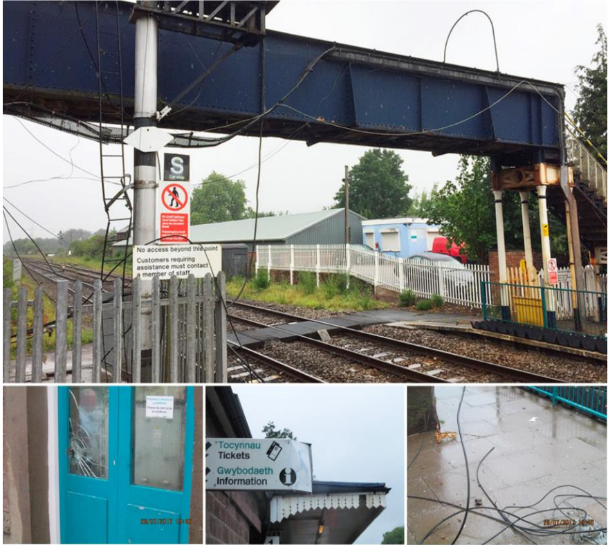
Fig 4. Detached cable tray running across the footbridge (to left of image)
