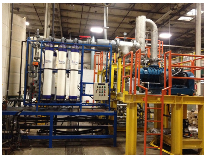
FIG. 7.5 25,000 L per day capacity AQUA SEP™ hybrid membrane distillation plant for sugar extraction and purification from MSW.
