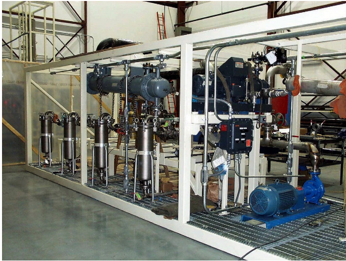
FIG. 7.8 20,000 L per day capacity AZEO SEP™ pervaporation plant for dehydration of solvents.
