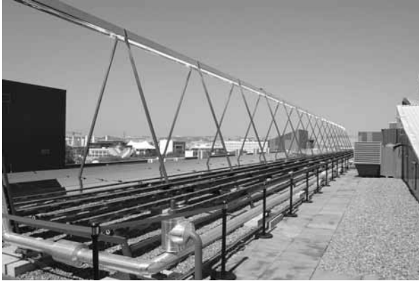
6.21 The third Industrial Solar project, built in 2007 in Seville, Spain, with an aperture area of 352 m 2 , length 65 m, pressurized water circuit at 16 bar, and operating temperature 180°C. The application was solar cooling with a double-effect absorption chiller (175 kW) (courtesy Industrial Solar GmbH, reproduced with permission).
