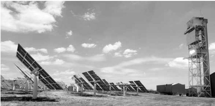
20.15 Solar tower facilities at the Plataforma Solar de Almería (PSA) in Spain (Konstandopoulos and Lorentzou, 2010).
