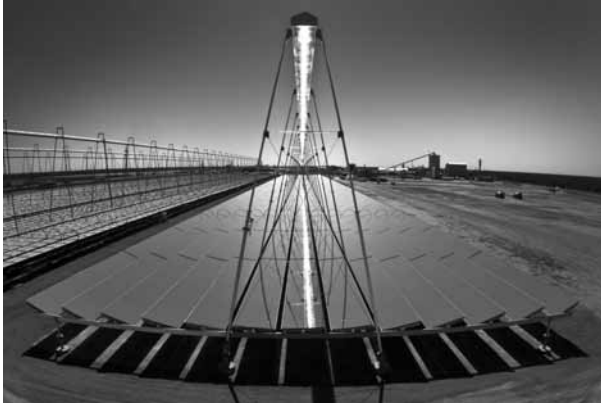
6.17 The fourth line at Kimberlina in operation. It differs from the first three lines in using 13 reflectors instead of ten, and in operating as a superheating line at 400°C (copyright Areva Solar, used with permission).
