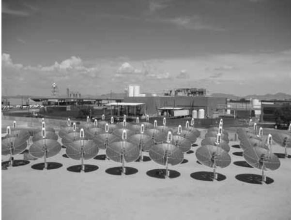
9.12 PowerDish installation in Yuma, Arizona 2010 by Infinia Corp. (Copyright: Infinia Corp.).
