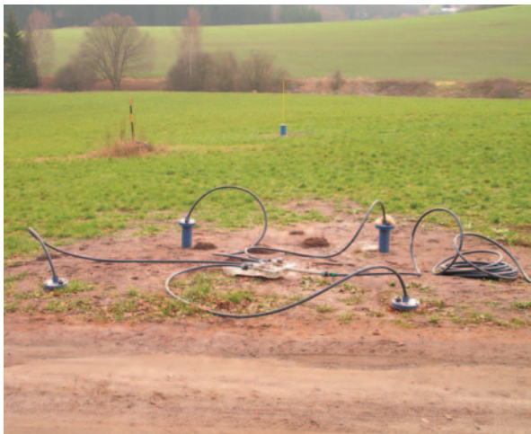
FIGURE 5 Injection wells at a contaminated site in the Czech Republic. © AQUATEST, CZECH REPUBLIC
