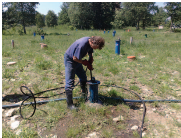
FIGURE 6 An nZVI slurry is pumped into the wells at a contaminated site in the Czech Republic. © AQUATEST, CZECH REPUBLIC
