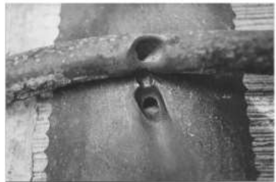
FIGURE 6.9 Pits in the galvanized water pipe that contributed to the erosion-corrosion of the gas line and the subsequent leak in a sewer main that caused the Guadalajara 1992 explosion [6]. (Courtesy of Dr. Jose M. Malo, Electric Research Institute, Mexico)
