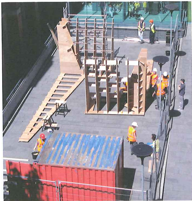
4 A workshop-based prefabrication sequence for component parts was predetermined by the sequence of assembly on site, and established batching for manufacture and delivery.
