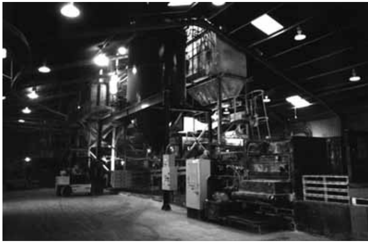
Figure 25: A typical milling facility to process Ball Clay.
