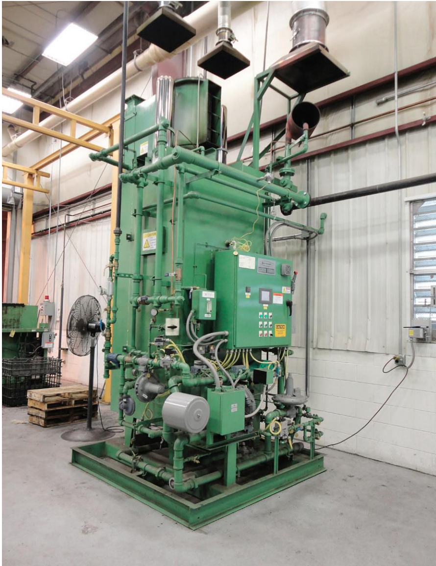
Fig. 2. Single-retort endothermic gas generator (courtesy of AFC-Holcroft)
