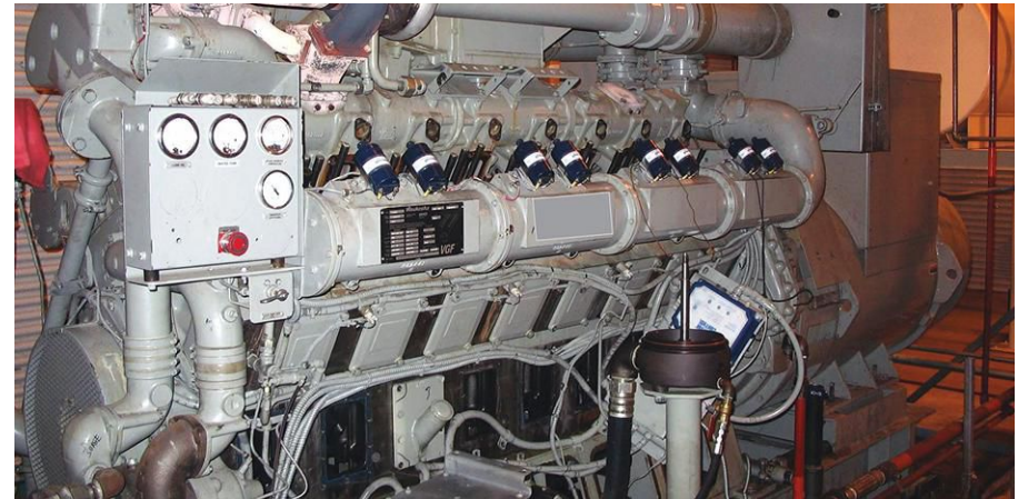
Fig. 1. Power generation diesel engine failure (photograph courtesy of Materials Engineering Inc.)
