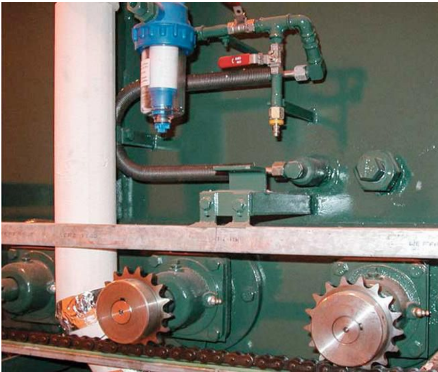
Fig. 2. Typical sample-port configuration on a continuous mesh-belt furnace
