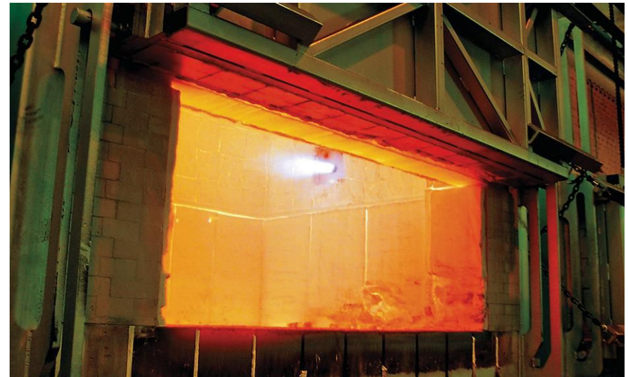
Fig. 2. Low-NO x burner in operation
