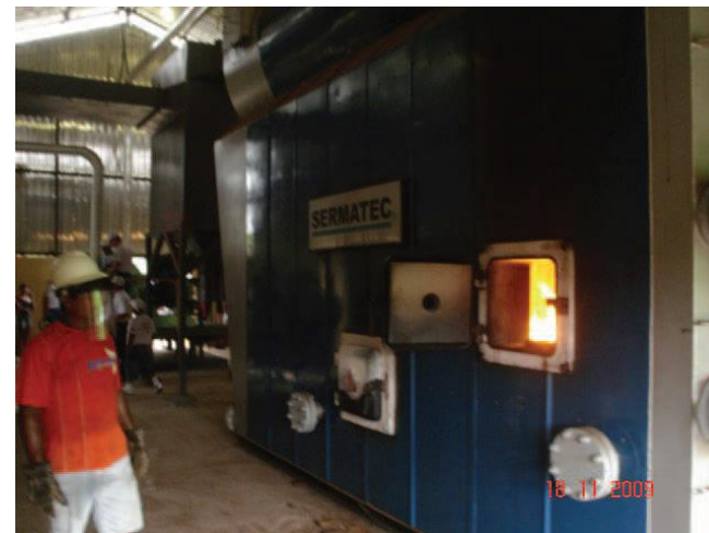
4. Start-up of the biomass-plant
