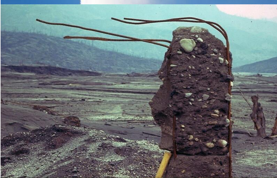
Building remnant in Francisco Leon destroyed by pyroclastic surges and flows during eruption of El Chichon volcano in Mexico 1982. Reinforcement rods in concrete bend in direction of flow.
