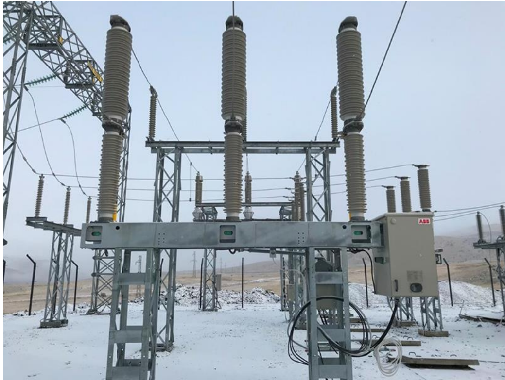
Figure 5-3: Site Substation for Power Grid Connection
