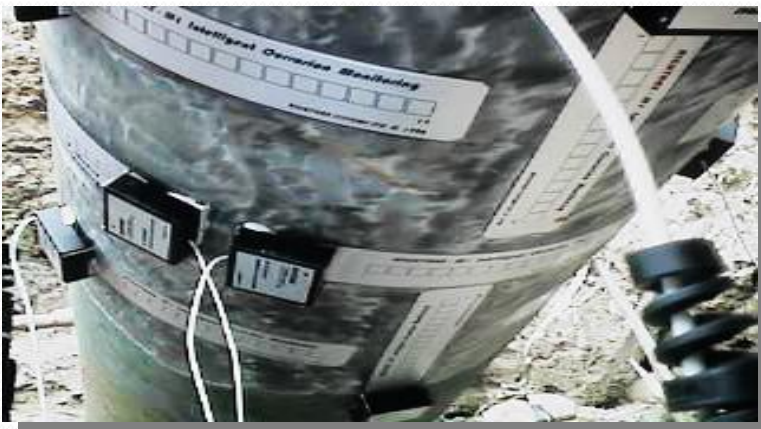
Multiple M1 Sensors fitted to subterranean Pipeline Prior to coating reinstatement and back filling
