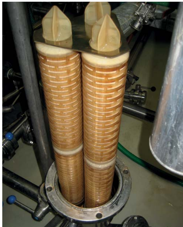
Figure 3: Thick dirt and iron deposits (filter cartridges).
