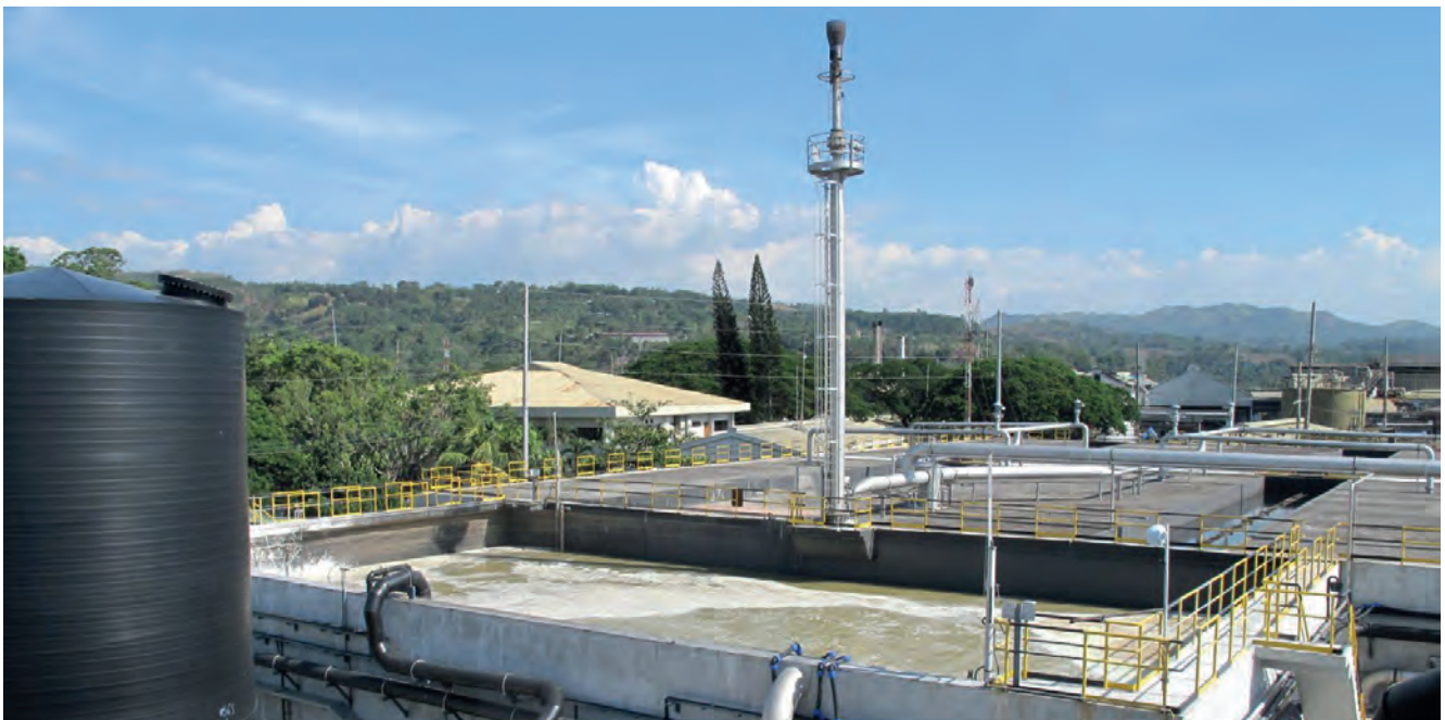
Green energy generators powered by biogas (methane) from waste water at Del Monte Philippines transform a problem into to a profit.
