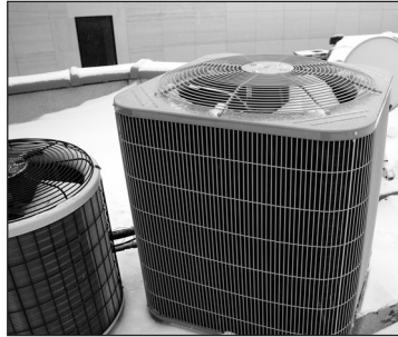
Air conditioning systems
