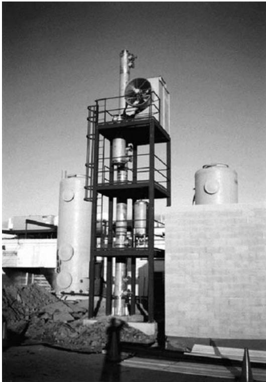
Fig. 32.16. Pollution control facility in Milford foundry, New Hampshire includes an adsorption tower. Gaseous emissions are introduced at the base of the treatment column, where a gas diffuser ensures that they are evenly distributed through the system. The gas then contacts purification liquid in the packing of sorbents (e.g. zeolite) in the absorption zone. A second diffuser ensures that the purification liquid is evenly spread. Source: Environ-Access, Inc. (1996). Environmental Fact Sheet, "Treatment of Air and Gas: Treatment of Gaseous Emissions through a Wet Scrubber—MESAR Environair Inc." (F2-03-96), Sherbrooke, Quebec, Canada.
