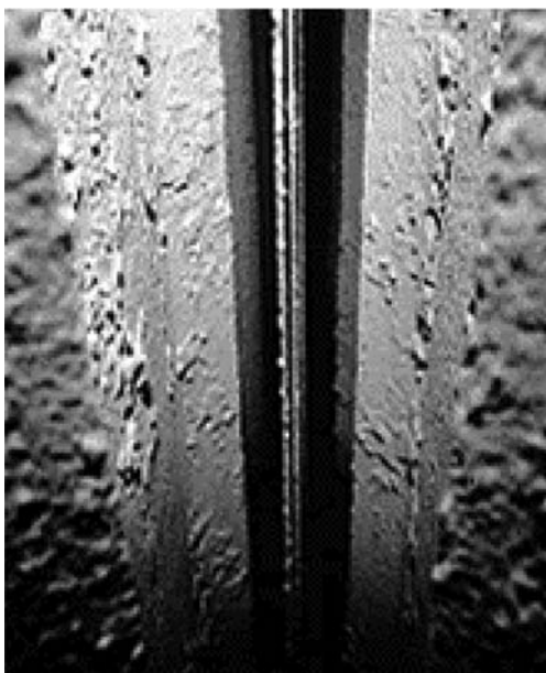
Fig. 32.7. View inward of a single gas passage through an electrostatic precipitator. The opening is about 20 cm.
