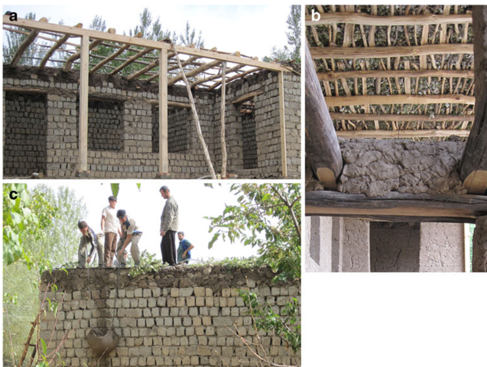
Fig. 2 Roof construction observed in rural Uzbekistan (Samarkand area, 2011). a Early stages of roof construction: wooden beams form the roof skeleton. b Later stages of construction: the wooden beams are covered by wood branches and leaves. c Final stages of construction: mud is plastered over the vegetal roof
