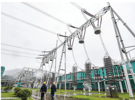
China's major ultra-high voltage transmission system is underway.
