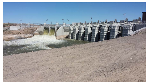
Fig. 7. Eight siphon-type Kaplan turbines. The units were installed by North Side Canal Company in Idaho, United States, in 2015. The site has a 6 m of head and a total of 1.28 MW installed capacity. (Used with permission of A Hansten of North Side Canal Company).
