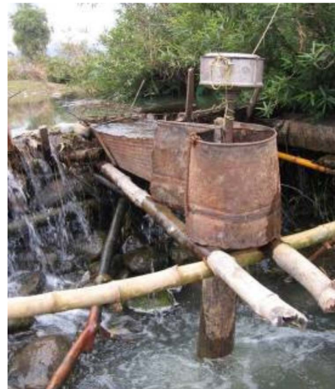
Fig. 6. Standing Pico-Hydro Unit in Khaivieng Village, Kham District, Xieng Khouang Province. (Used with permission of M Smits [27]).
