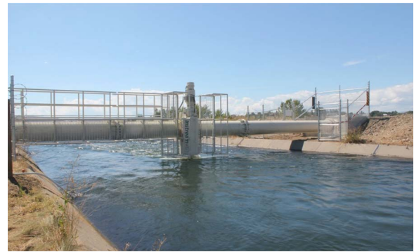
Fig. 2. Structure to support testing of a turbine that produces electricity from flowing water. Instream Energy Systems of Vancouver, B.C., built this structure over the Roza Canal in the Yakima Basin in Washington State to support testing of a turbine that produces electricity from the flowing water. (Used with permission of Instream Energy Systems Corporation).
