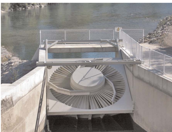
Fig. 9. A 410-kW very-low-head turbine unit in the Tarn River, Millau, France. (Used with the permission of M.J2 Technologies S.A.S.).
