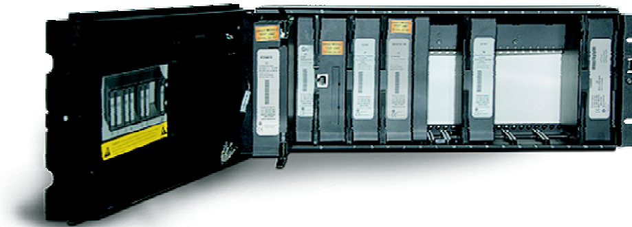
Figure 10-4: Modules inside relay with front cover open (enhanced faceplate)
