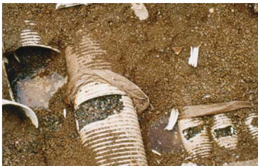
Fig. 6 Drainage pipes filled with the material from the gravel and sand fill layer
