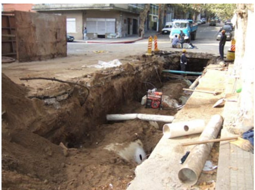
Fig. 20.22 The sub-surface of any street can be a complicated environment, creating uncertainty in full construction costs.
