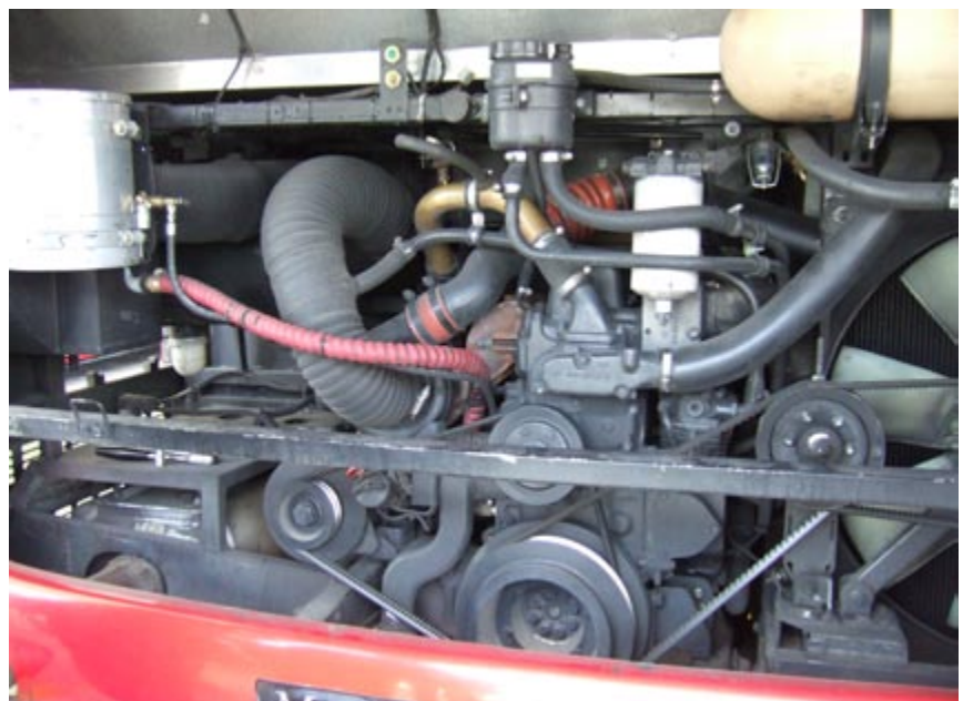
Fig. 12.37 Diesel technology has a long operational track record, and thus the technology's robustness and maintenance requirements are well know.
