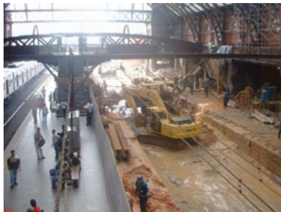
Fig. 2.27 and 2.28 An initial BRT corridor may take 12 to 24 months to construct (left photo); by comparison a typical underground or elevated rail system will require from three to ten years (right photo).
