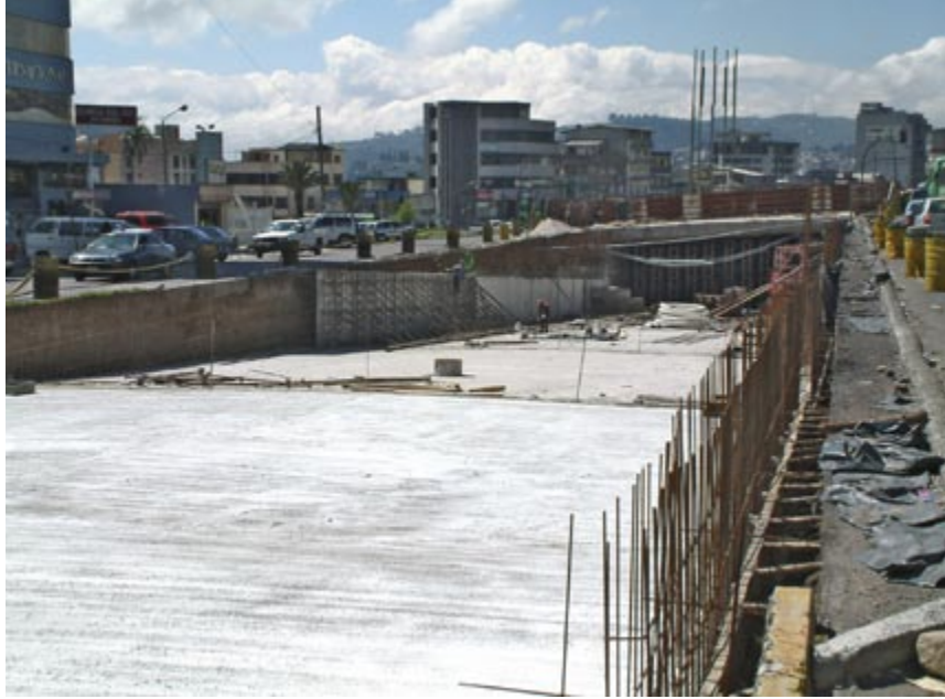
Fig. 20.32 Re-routing traffic around intersections that are under heavy construction can be particularly challenging.
