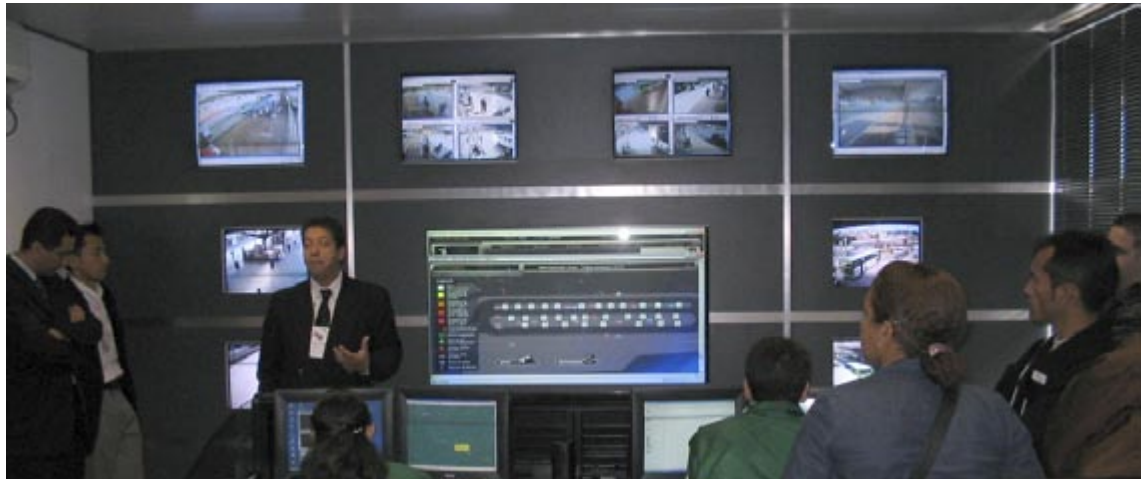
Fig. 11.122 A distributed control centre at the Perituba Terminal in São Paulo. Photo by Dario Hidalgo
