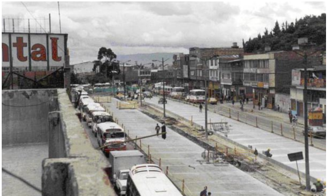
Fig. 20.33 The disruption to traffic and businesses during Phase I construction of TransMilenio did receive some criticism. More mitigation measures were subsequently applied in Phase II.
