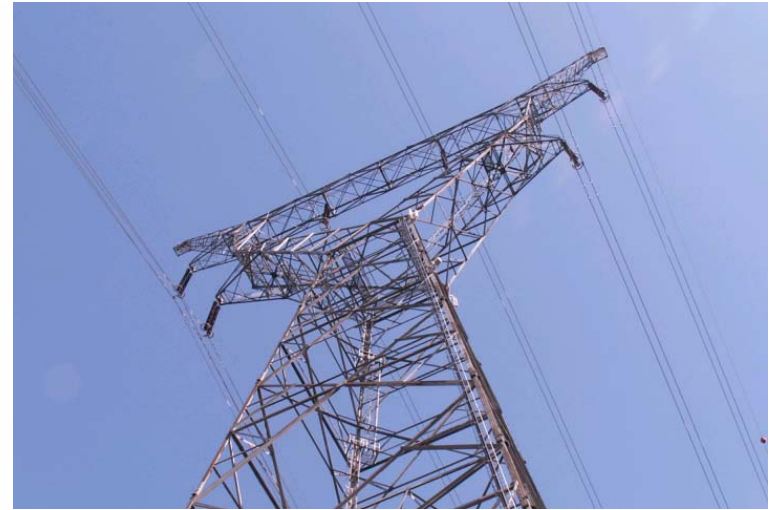
High Voltage Power Systems
