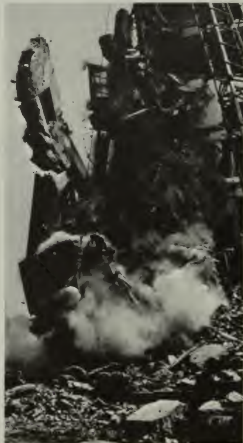
Fig. 3-22 A 1,350-kg steel ball swung by a crane against the walls of a condemned building. What happens to the momentum of the ball?
