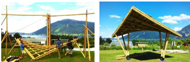
Figure 12 a and b: a: Guadua hyper grid ready to be lifted, note that the limited rise allows to work on the joints without scaffolding. b: finished hyper at the Base Habitat workshop
