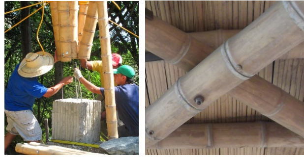
Figure 3 a and b: connection of guadua poles to foundation (left) and interconnection of guadua poles (right)
