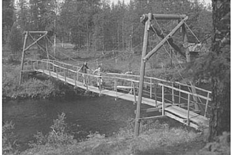
An example of a fairly basic suspension bridge over a river in Finnish Lapland. The main cables should be tightened to prevent the sag in the middle and to reduce the swing and bounce experienced when crossing the bridge.
