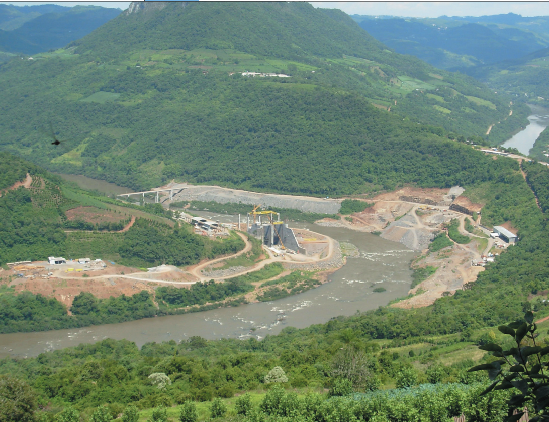
Figure 1: Construction of a small hydropower plant on Antas river, Rio Grande do Sul, Photo: Luis E. Sánchez
