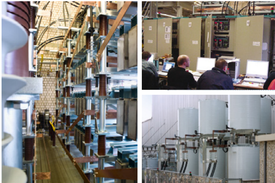
Fig. 22: 30 MW Hardware Functional Tests
