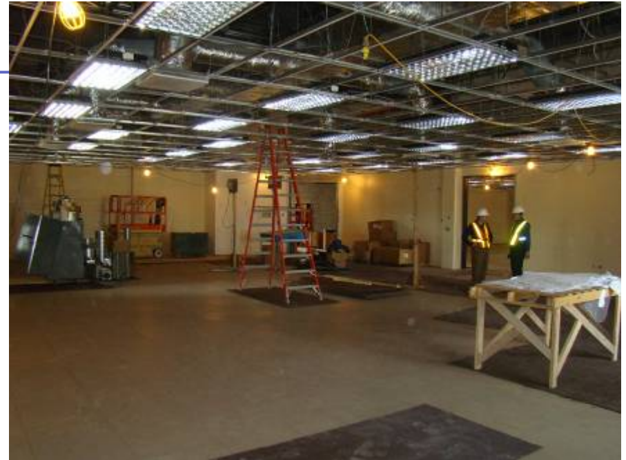
June, 10 – Control Room – Second Floor
