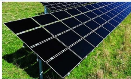
Thin film solar panels
