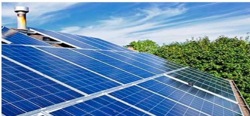
Polycrystalline solar panels
