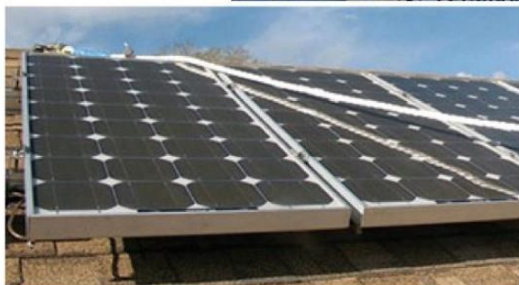
Mono-crystalline solar panels
