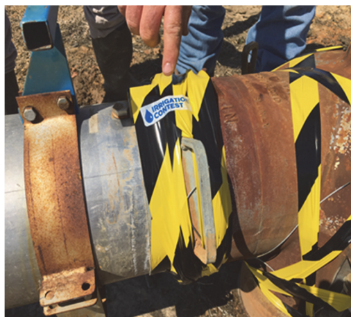
Figure 1. Sealing a flowmeter to prevent tampering with the measured irrigation amounts.
