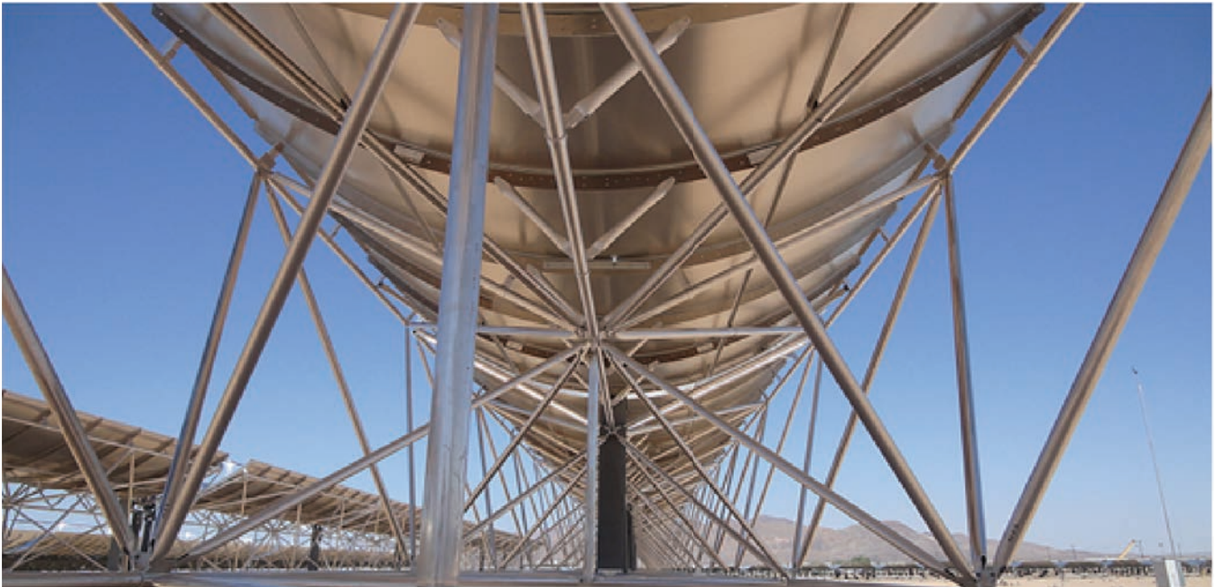
Figure 32: Detail of SkyFuel collector structure
