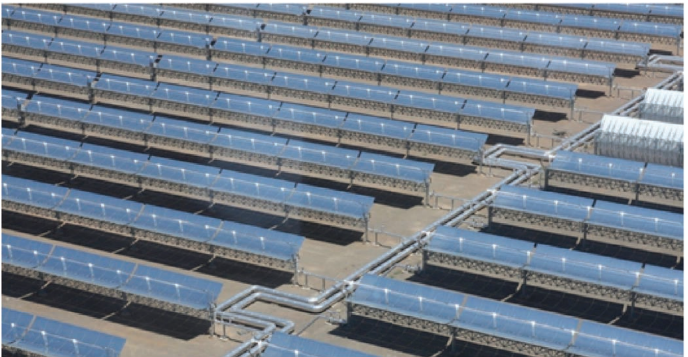
Figure 16: Parabolic Trough collector field with header piping
