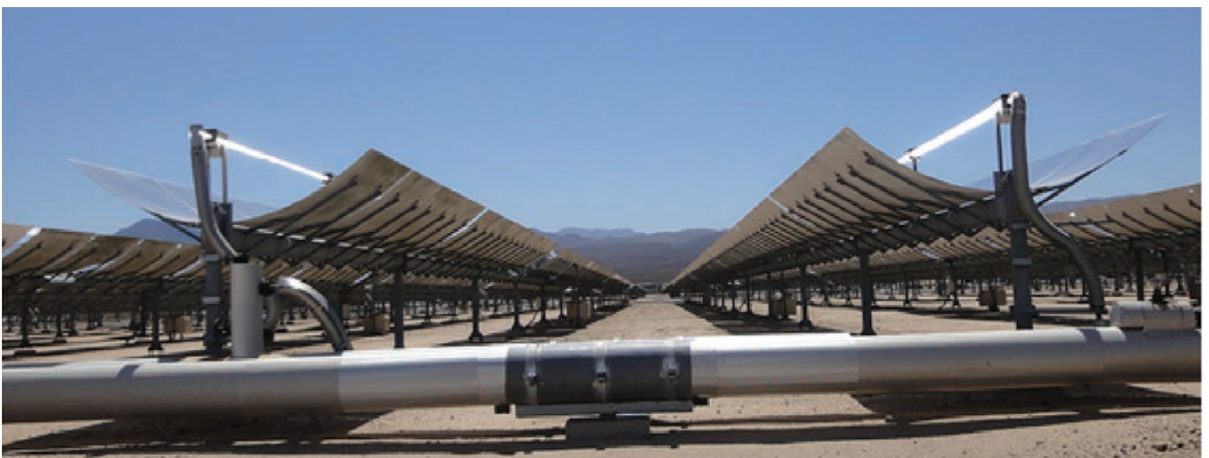
Figure 17: LS-1 collectors at SEGS II, Daggett (Photo: G. Weinrebe)
