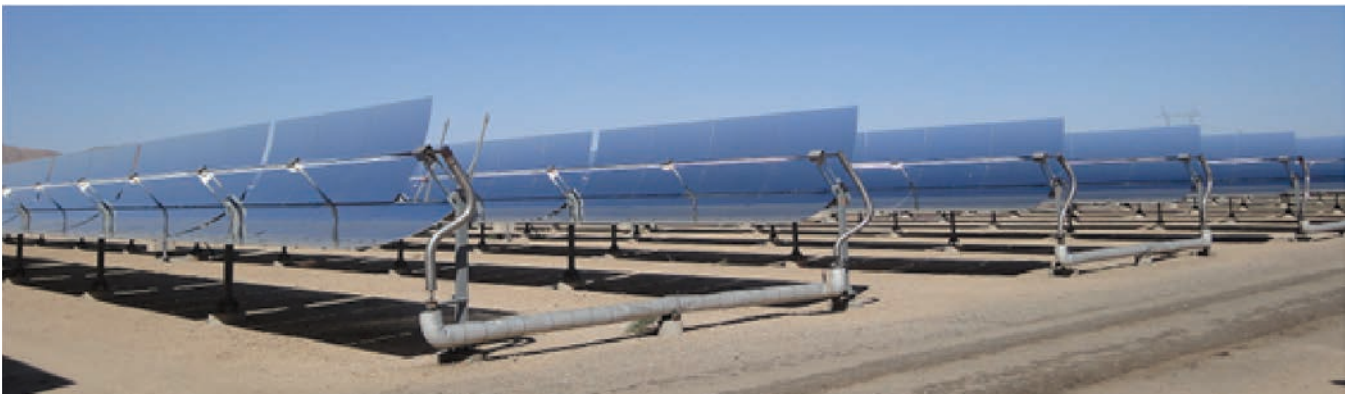
Figure 3: SEGS II plant at Daggett, CA
