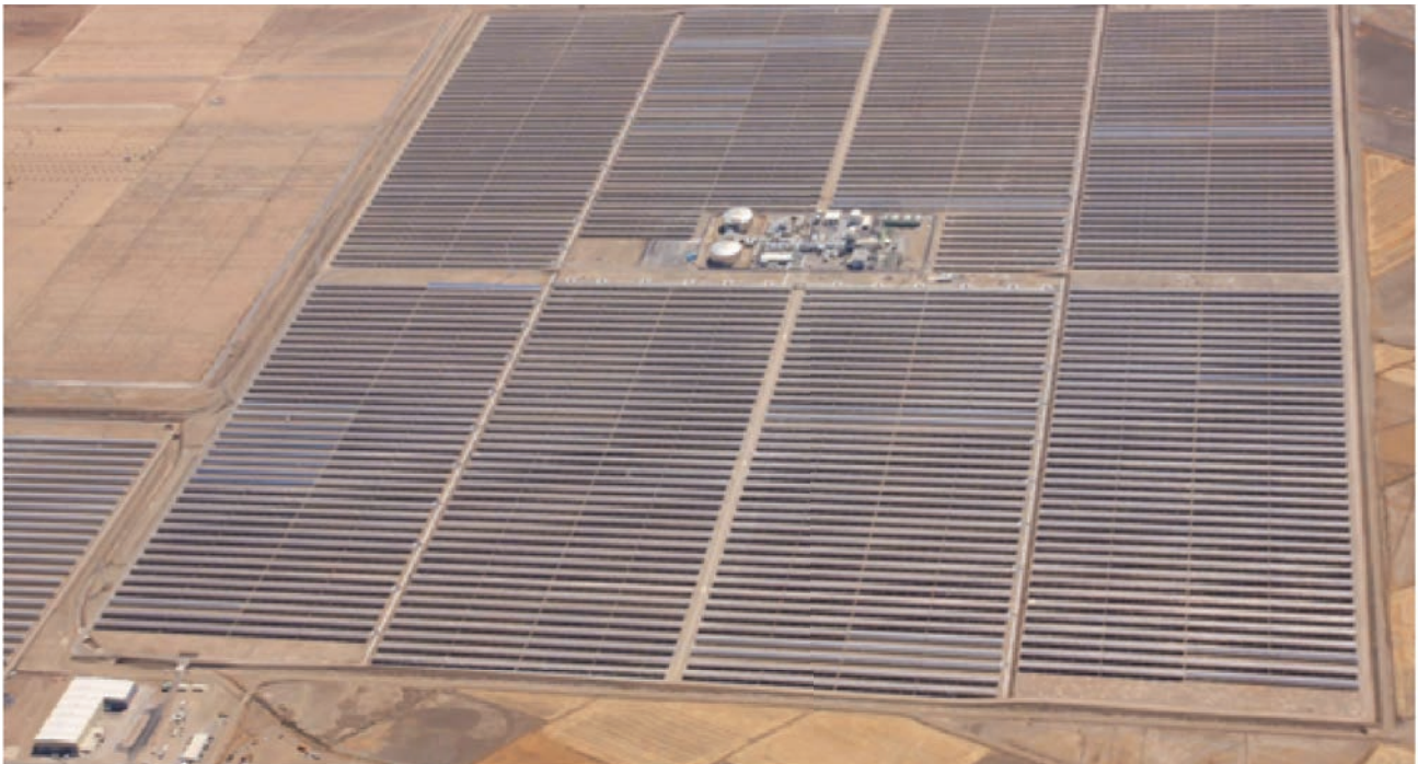
Figure 2: Solar Collector Field with power block and heat storage tanks in the center (50 MW Andasol plant in Spain)
