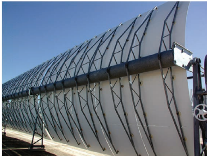
Figure 18: LUZ LS-2 parabolic trough collector [12]
