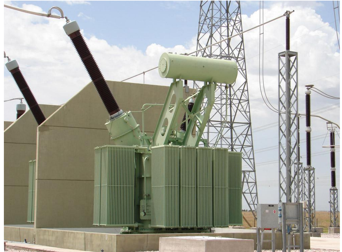
Reator shunt monofásico a óleo, 500 kV, 50 MVA
