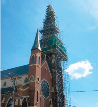
Fig. 4 The scaffolding required to renovate this church is similar to the ghost lines, centerlines, planes, and other reference geometry used in sketching.
