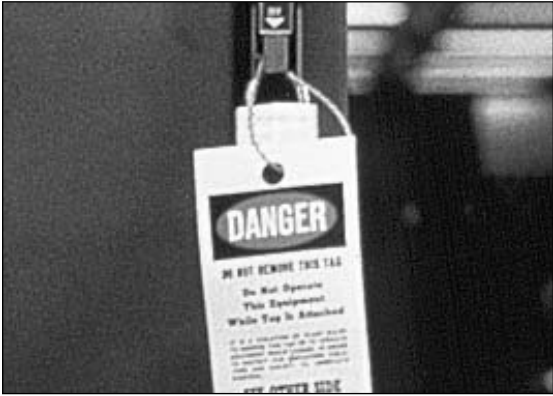
Power should be shut off and controls locked before inspecting
