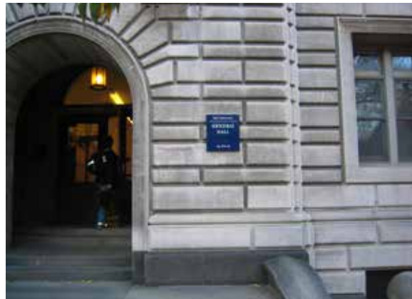
Sign placed high to avoid matching coursing lines.
