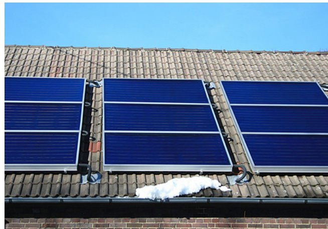
Solar water heater (left)
