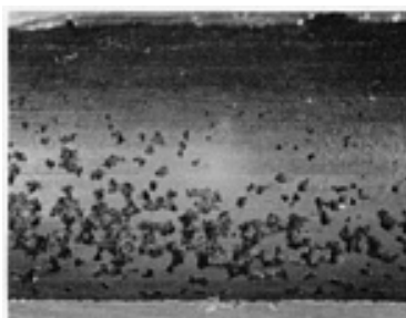
Fig. 11 Internal surface of carbon steel pipe section damaged by cavitation
