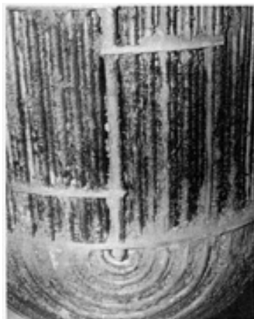
Fig. 5 Fouled heat-exchanger tube bundle
