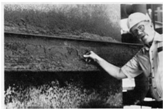
Fig. 6 Delamination of plain carbon steel due to \text{SO}_2 + ash deposit outside the boiler area of a coal-fired power plant. Courtesy of D.M. Berger, Gilbert/Commonwealth
