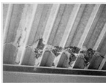
Fig. 1 Corroded steel formwork on the ceiling of a parking garage. The seams in this corrugated structure act as condensation traps and lead to wet atmospheric corrosion. Courtesy of R.H. Heidersbach, California Polytechnic State University
