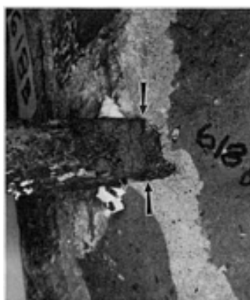
Fig. 15 Severe corrosion and cracking (arrows) on wall tie
