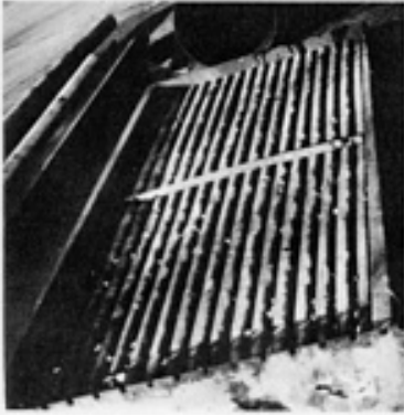
Fig. 4 Corrosion on air conditioner cooling fins
