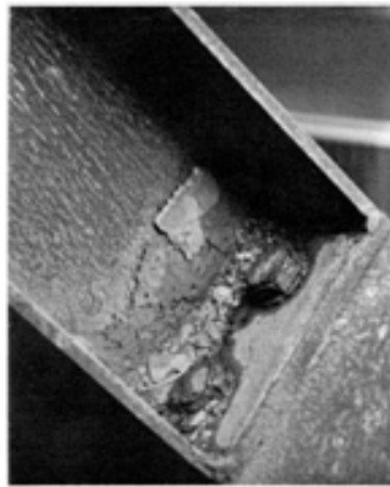
Fig. 11 Heavy corrosion scale buildup on structural members of weathering steel at a pocket where water could collect and stand
