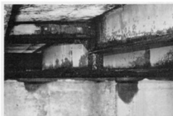
Fig. 5 Corroded regions on a painted highway bridge. Courtesy of R.H. Heidersbach, California Polytechnic State University
