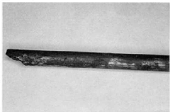
Fig. 20 Pitting corrosion adjacent to fracture on failed posttensioning wire
