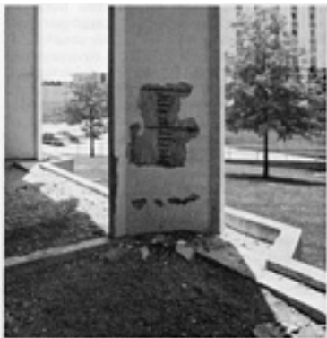
Fig. 12 Corrosion-induced spalling of overlying concrete on reinforced columns. See also Fig. 13
