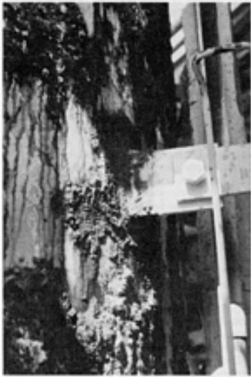
Fig. 8 Corrosion around the ladder clip of a gas-processing column. The column was painted with an inadequate protective coating (0.05 mm, or 2 mils, of epoxy) that could not prevent corrosion near the moisture entry points.
