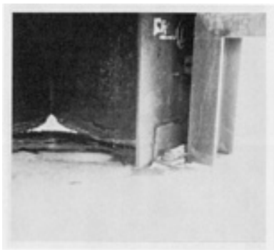
Fig. 25 Formation of lamellar rust due to moisture wicking upward from beneath concrete pad. The buried portion must be painted.
