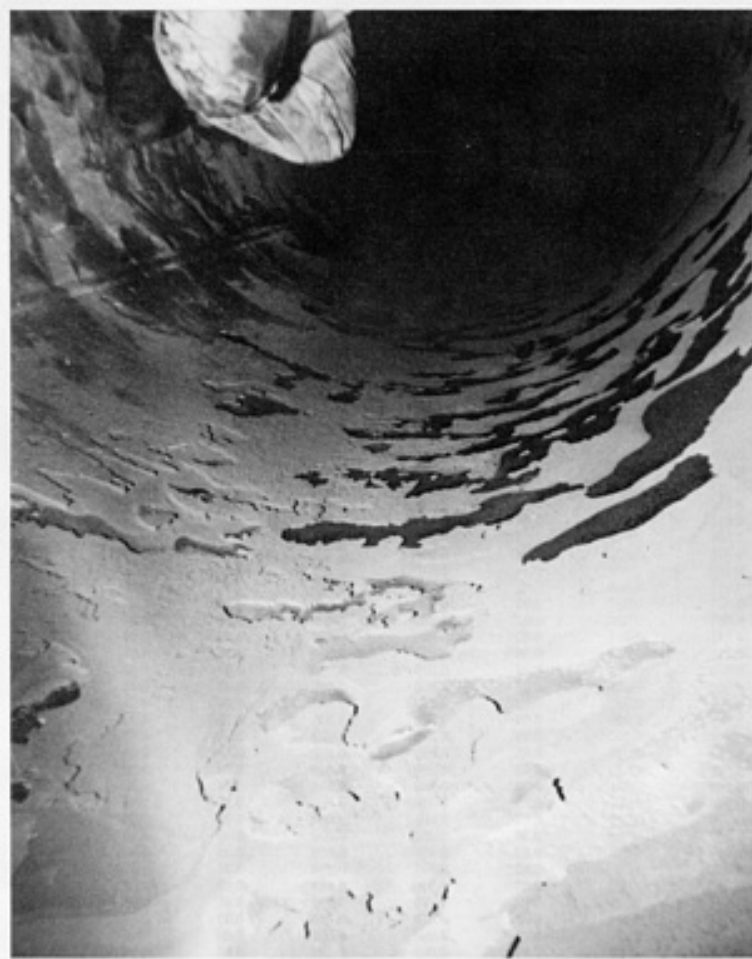
Fig. 70 Erosion-corrosion damage in wet steam piping. Source: Ref 135
