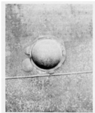
Fig. 4 Debonded organic coating near a high-silicon cast iron button anode
