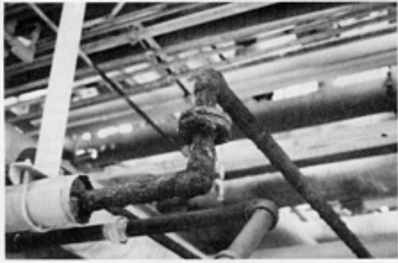
Fig. 10 Heavy general corrosion of a steel line insulated with cellular glass and aluminum outer jacketing. The line is at ambient temperature except when it is used to vent hydrocarbons. Temperature then decreases, causing moisture condensation, followed by warming to ambient temperature and slow corrosion. The line was replaced after 11 years of service.
