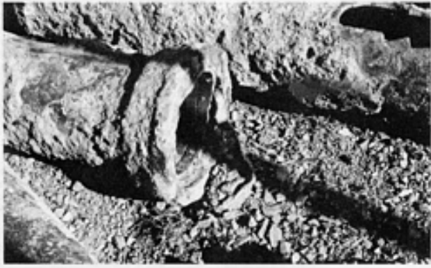
Fig. 5 Corrosion failure of an underground cast iron pipe
