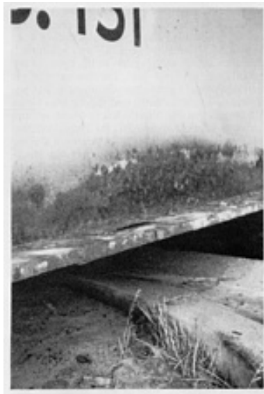
Fig. 4 Corroded weathering steel highway bridge girder. Courtesy of D. Manning, Ontario Ministry of Highways and Communications
