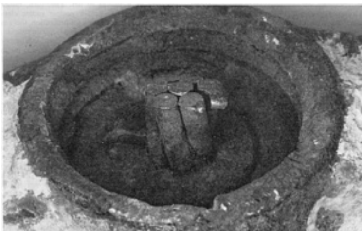
Fig. 18 Corrosion of posttensioning anchorage. Note severe corrosion at the two wedge halves
