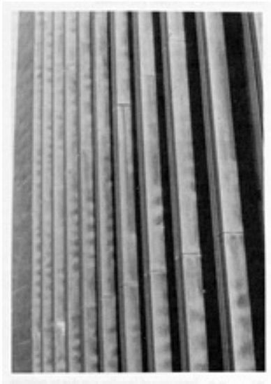
Fig. 28 Clad columns with less than 18-gauge cover, resulting in oil canning
