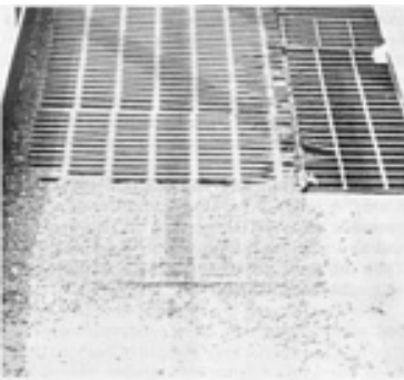
Fig. 3 Cracking and spalling of a concrete floor
