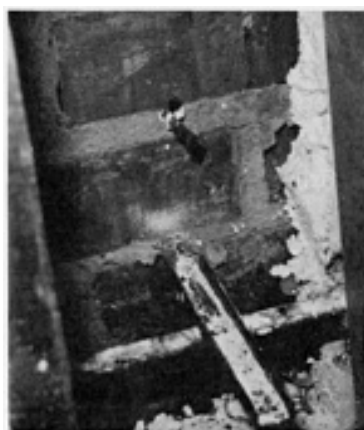
Fig. 14 Unconventional masonry tie constructed from flattened C-channel and bent to enter the brick core
