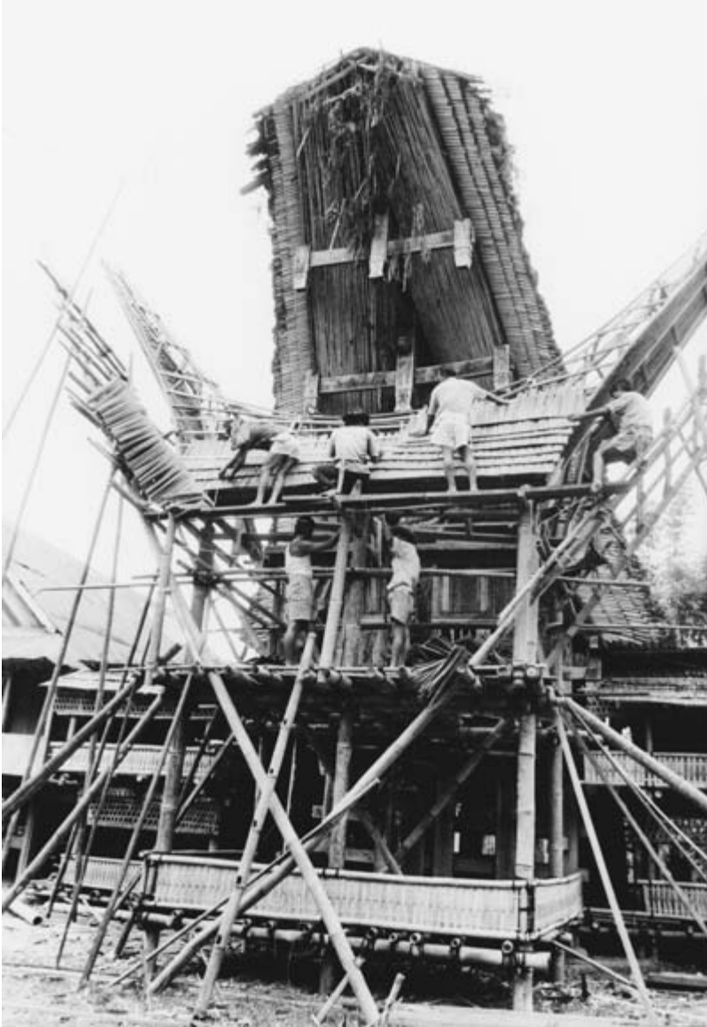
3.1 Toraja villagers often use their carpentry skills in communal labor to build the temporary structures used in rituals. Here villagers are preparing for a funeral by constructing, in front of the deceased's house of origin, a tower to hold the corpse during the final days of the mortuary rites. Hundreds of guests will be housed in temporary two-story shelters built around the house yard. Tana Toraja, Sulawesi, Indonesia, 1996. Photo: Roxana Waterson.
