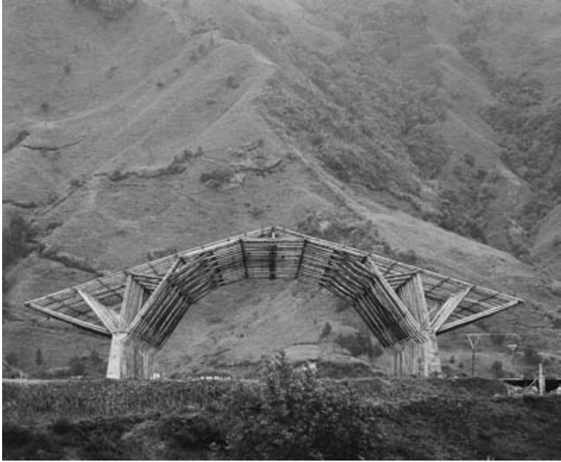
3.10 Factory hall under construction in Pensilvania (Colombia), an experimental large-scale design in bamboo by Colombian architect Simón Vélez, 1993. Photo: Günter Pauli, ZERI Foundation.
