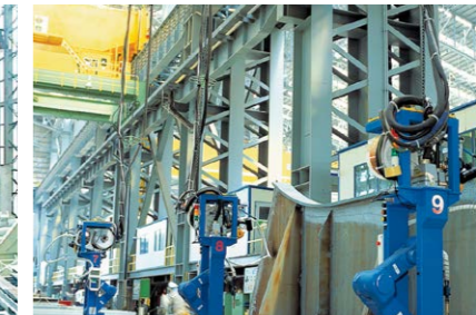
Automatic welding robots operated by an off-line program (controlled directly from the main yard computer) ensure high-quality welding.
