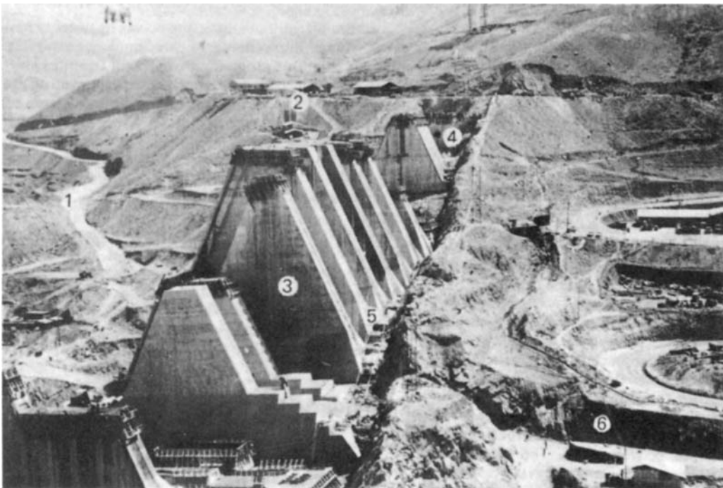
Fig. 15.14 Concrete buttresses of the Farahnaz Pahlavi Dam. 1 Access to site. 2 Future top water level. 3 Buttresses. 4 Excavation for key into hillside. 5 Spread base for low bearing pressures. 6 River channel. (Photograph by Sir Alexander Gibb and Partners.)
